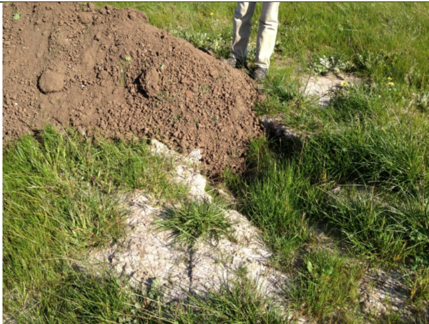
PLATE 10 Topsoil brought to the location of the previous test-pit and awaiting filling.
