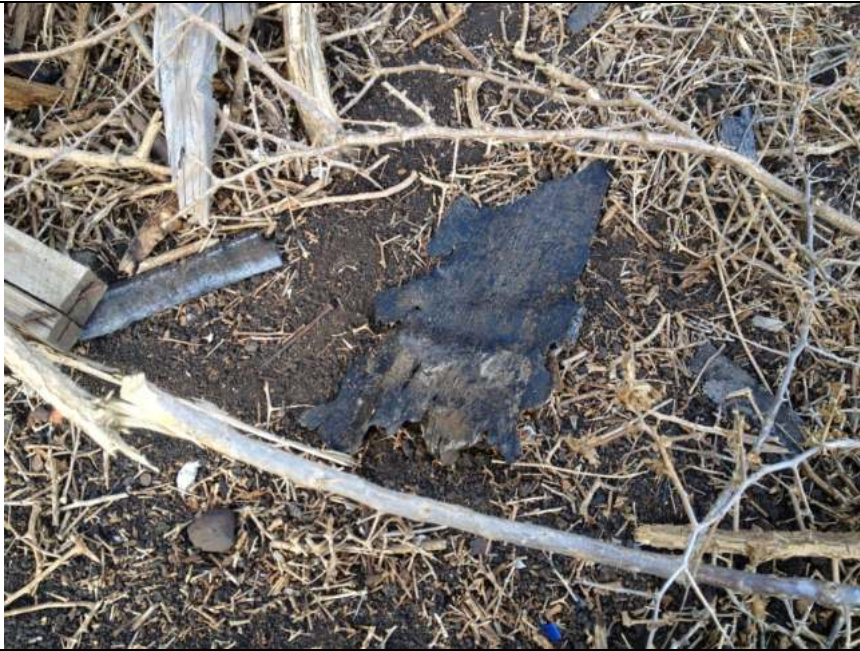
PLATE 3. Bituminous roofing material found to contain asbestos.
