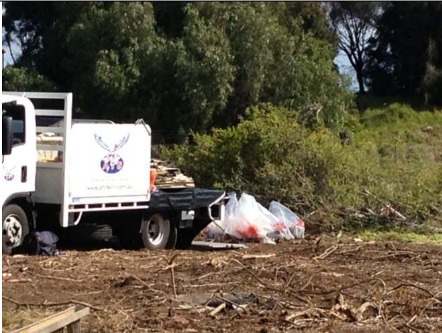
PLATE 5 Double bagged asbestos awaiting removal from site.
