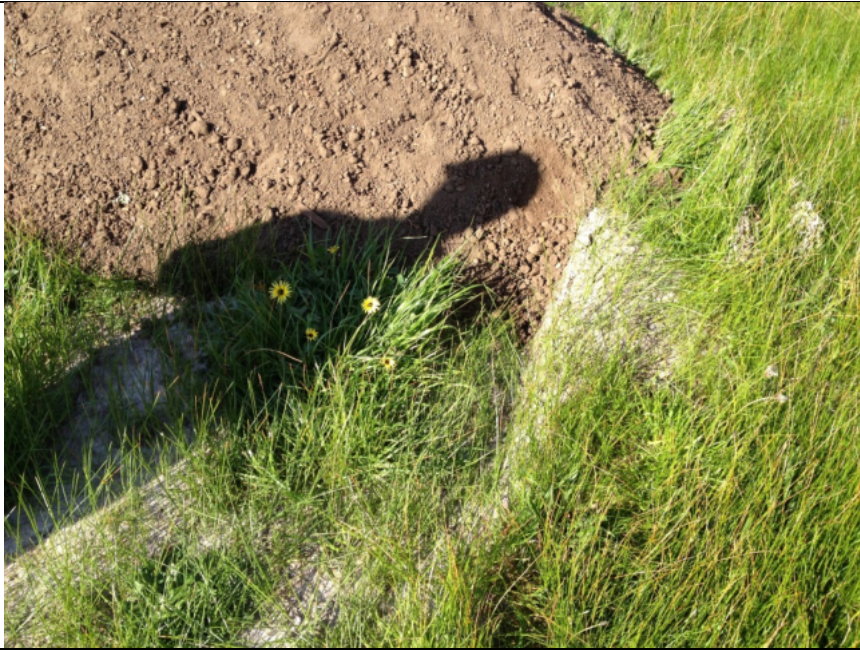
PLATE 11 Topsoil brought to the location of the previous test-pit and awaiting filling.
