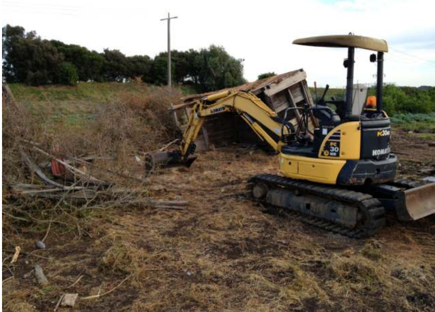
PLATE 1 Looking north at the area of removed farm buildings along the western boundary.
