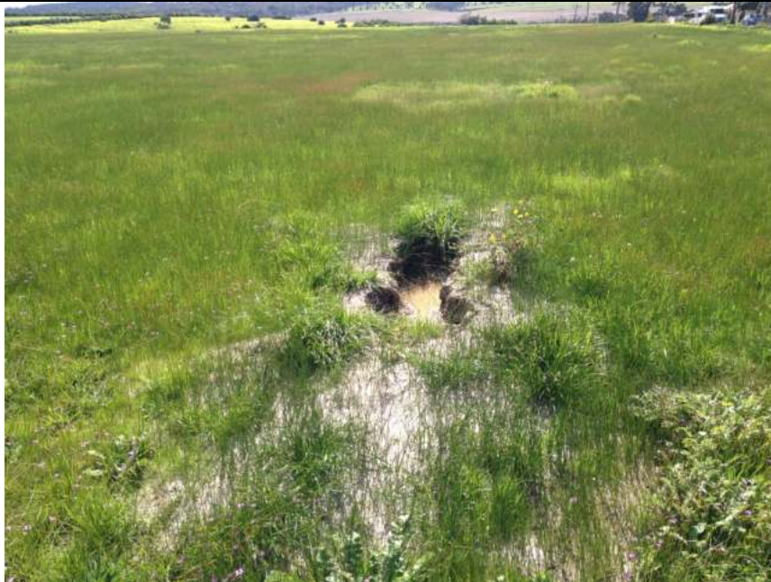
PLATE 12 Previous test-pit that has been backfilled and subsided.
